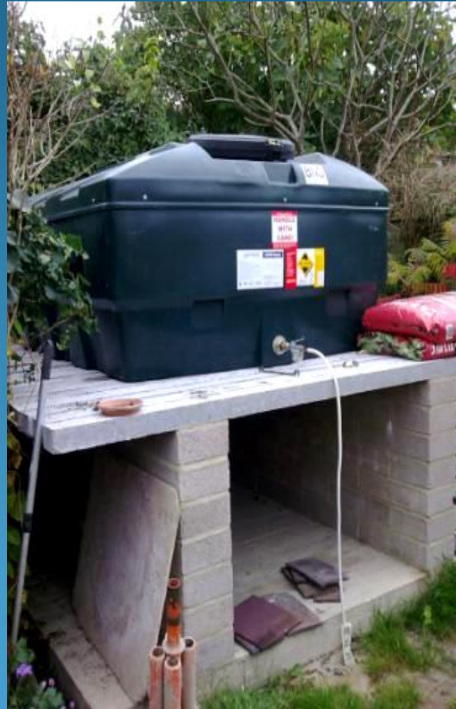
Oil tank above flood height
